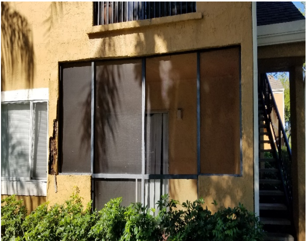
Photograph 3: Unit 104. Shoring required
