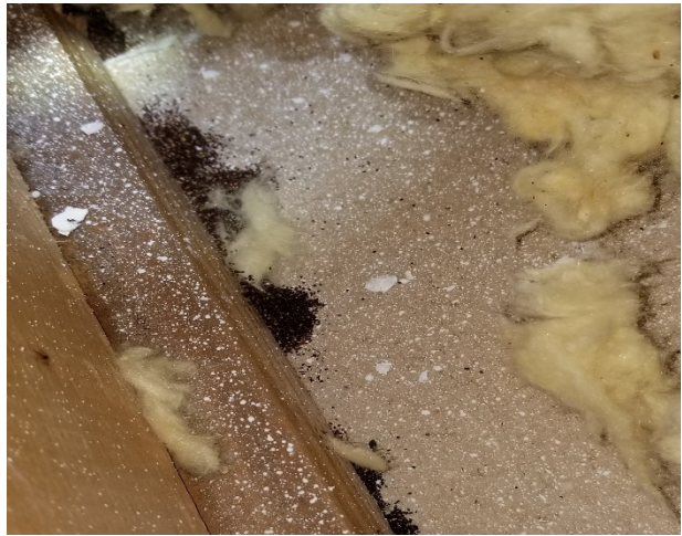
Photograph 8: Unit 202. Termites infestation in the attic
