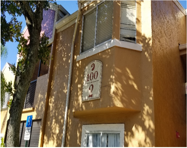
Photograph 1: Building elevation. Balcony wall cracking
